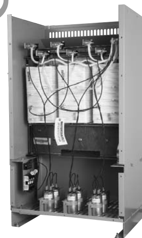
Guard II Transformer, (front panel removed)
