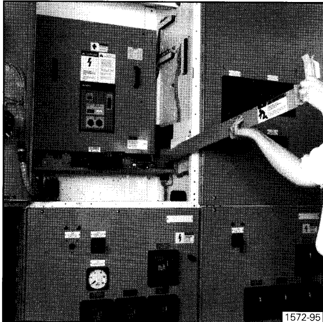
Figure 39. Use of Extension Rails for Removal of Circuit Breaker from Upper Compartment
