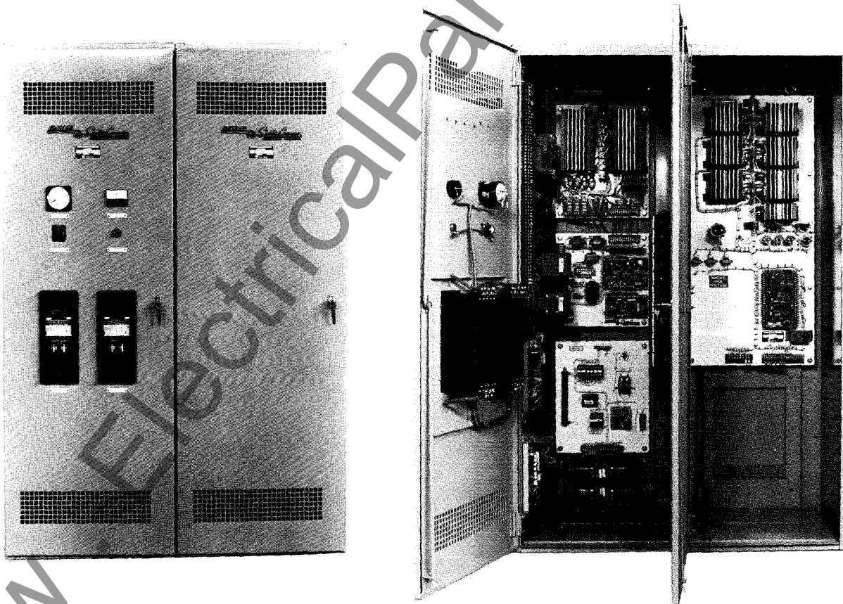
FIGURE 2 – ESS IN CUBICLE
