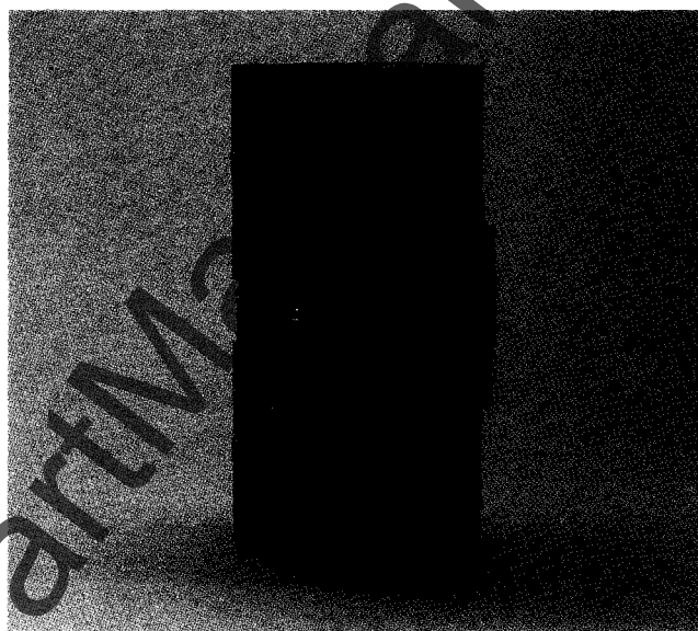
Fig. 5.2 Shunt trip leads run behind back of panel-mounted breaker
