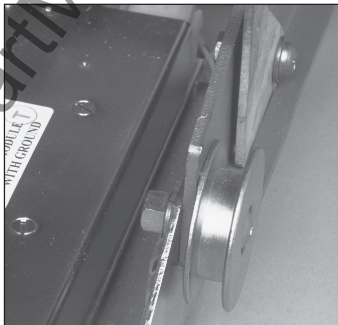
Fig. 15 Auxiliary CT Mounted in the Breaker
