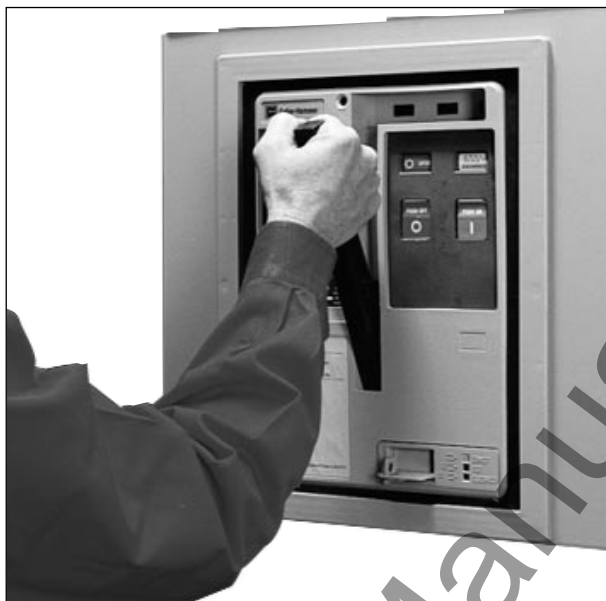
Magnum Circuit Breaker Being Manually Charged
