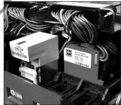
Figure 3 Shunt Trip Switch Installed
