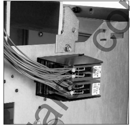
Figure 15 Cell Switches Mounted on Cassette
