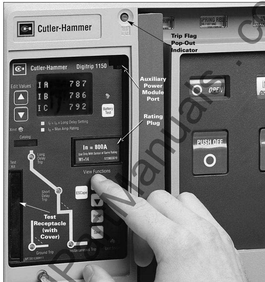
Digitrip RMS 1150 Programmable Trip Unit Installed
