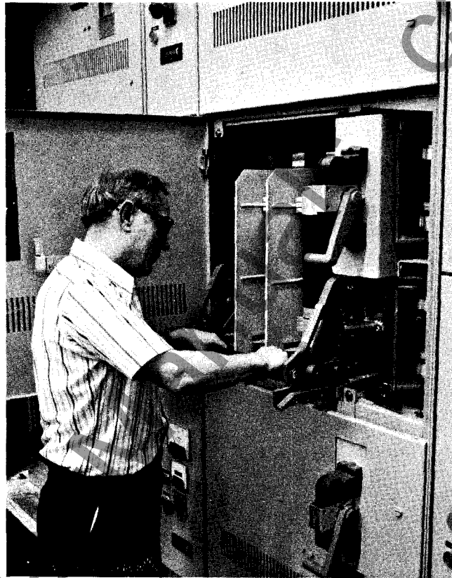
Fig. 45. Pulling on contactor positioning handle.
