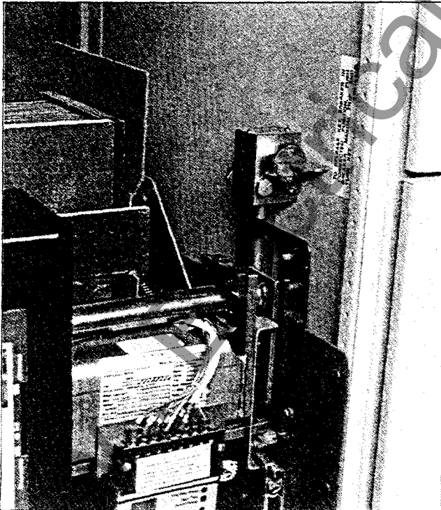
Figure 12. Key Interlock Mounted in Circuit Breaker Compartment
